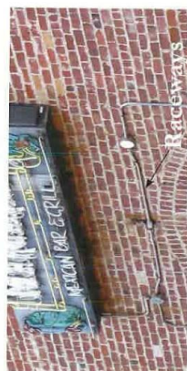
Exposed electrical raceways are not allowed.
