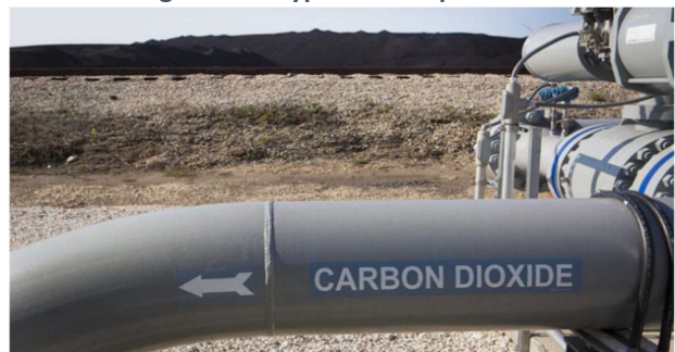
Figure 17 – Typical CO 2 Pipeline 36
