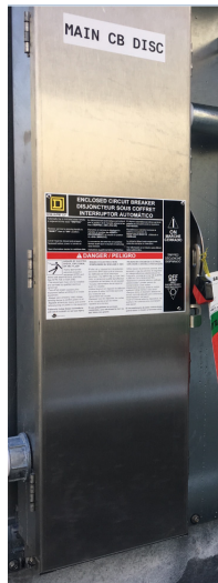
Figure 31. Externally mounted disconnect with circuit breaker
