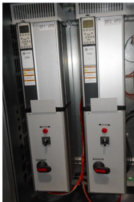
Figure 32. Drive mounted disconnects
