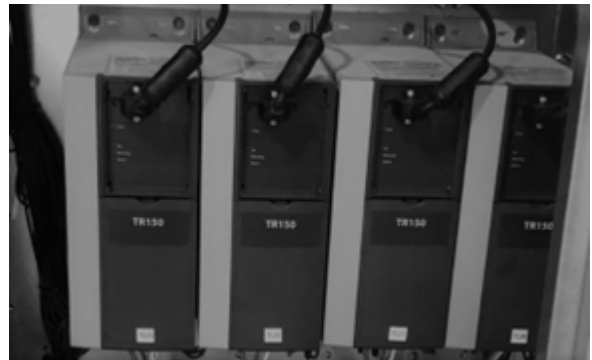
Figure 50. Trane TR150 VFDs
