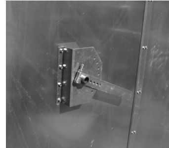
Figure 45. Handle to control linked dampers
