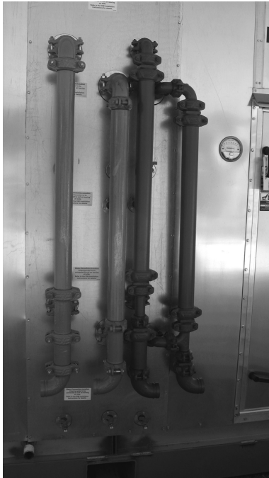
Figure 39. RSAU0050F1 piping manifold
