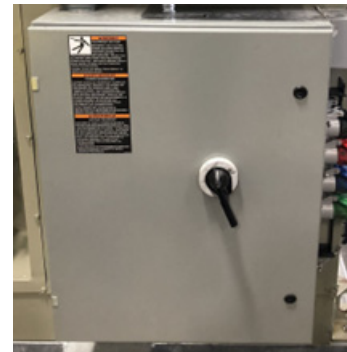
Figure 34. Externally mounted circuit breaker
