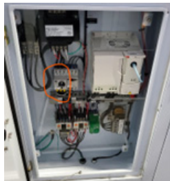
Figure 26. Internally mounted circuit breaker
