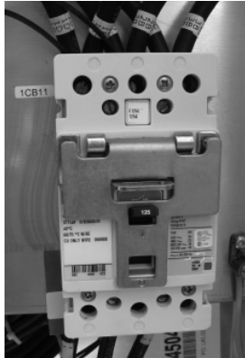
Figure 30. Internal circuit breaker
