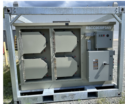
Figure 46. Discharge air flex duct connections
