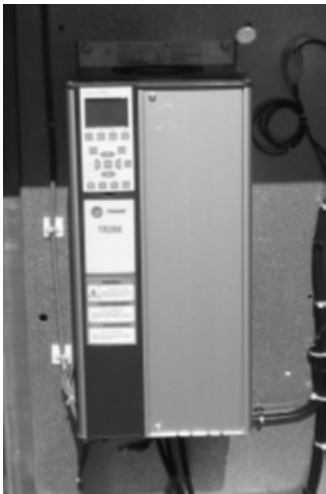
Figure 48. Trane TR200 VFD
