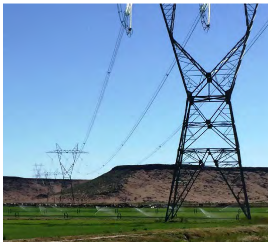
500-kilovolt (kV) transmission line near Melba, Idaho
