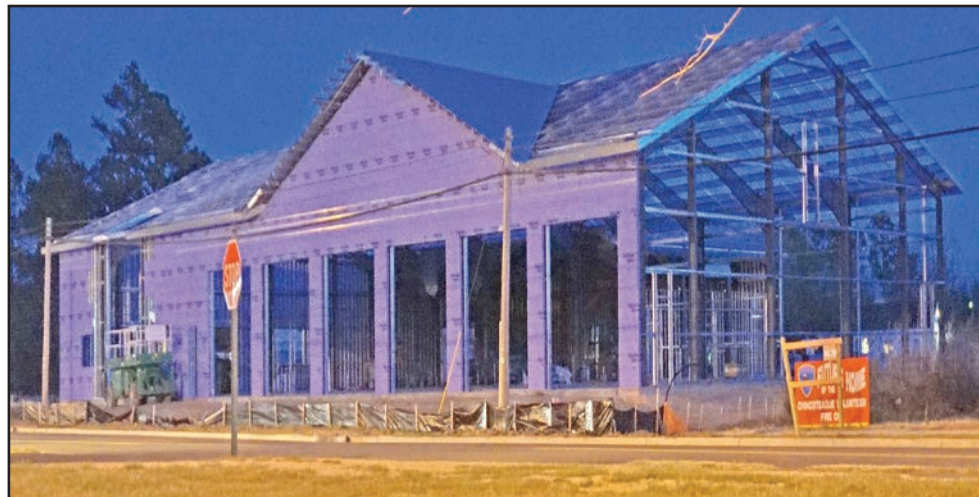
Chincoteague town council donated more than $30,000 in water line connection fees to help with the fire company's new firehouse construction.
