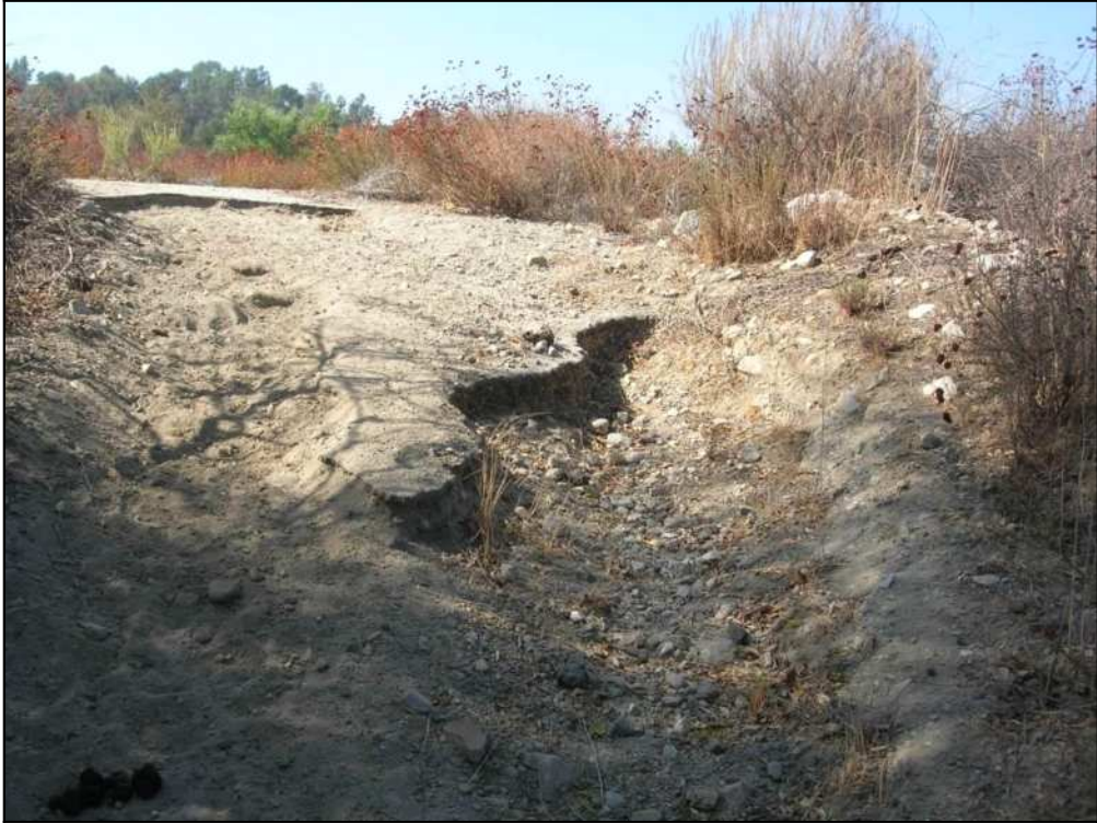
Figure 5. Erosion near Cottonwood Avenue entrance.
