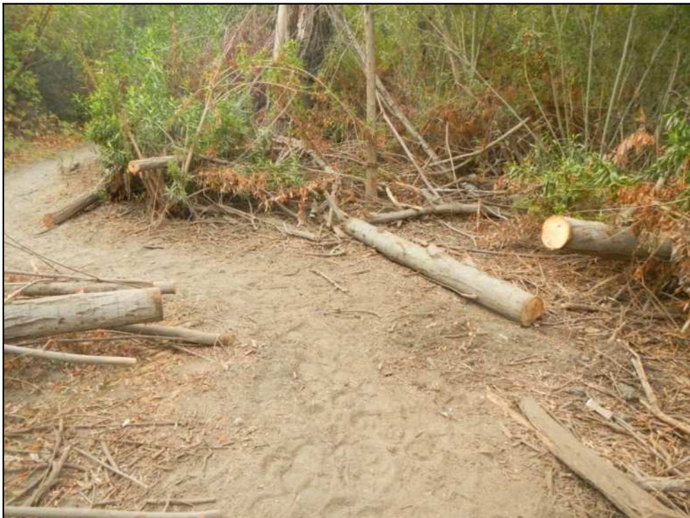
Figure 6. Cleared trail after tree removal was conducted on the trail south of the Tujunga Ponds.
