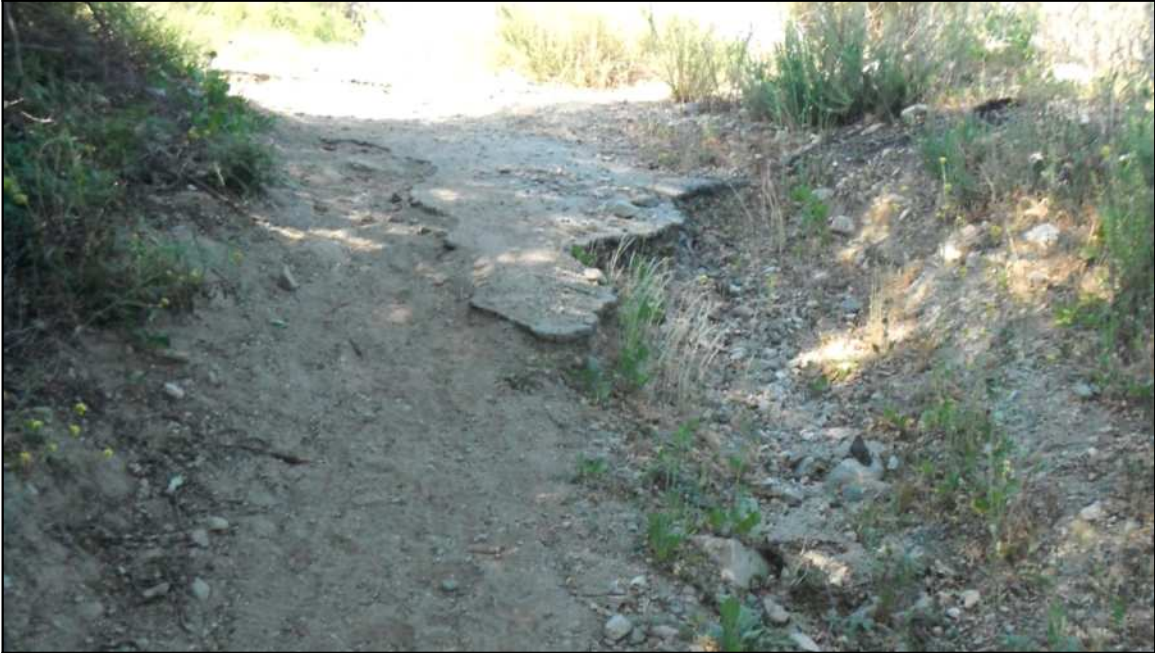
Figure 1. Trail Erosion Northeast of Cottonwood Gate.
