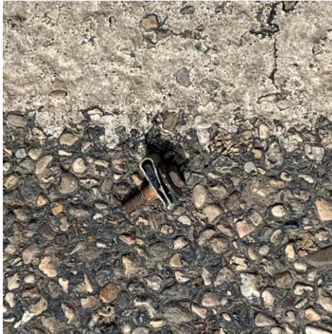
Figure 3: Bolt along fog line
