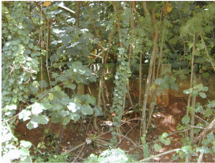
Photo view of the bottom of the ditch at the proposed culvert crossing.
