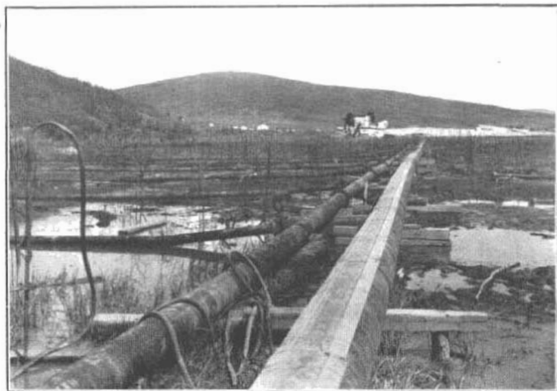
B. THAWING FROZEN GROUND WITH COLD WATER IN PREPARATION FOR DREDGING ON GOLDSTREAM, FAIRBANKS DISTRICT.
