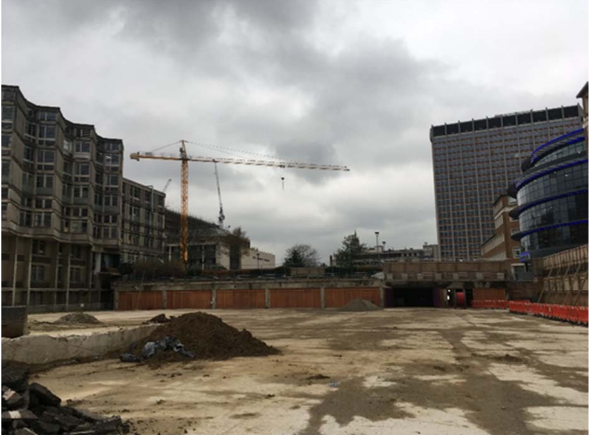
Photo from basement level within the site (Looking west towards the Annexe building (left) Fair Field public realm podium (centre) and College building (right))
