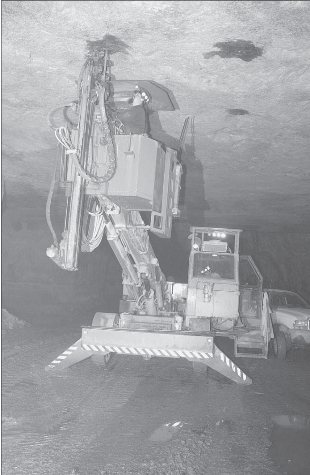
Donny Collins uses a Fletcher roof-bolter to bolt the 42-inch-thick roof (caprock) in the East Fairfield Coal Co. underground limestone mine in Mahoning County. Two rows of bolts are normally placed down the center of the entry, but the pattern will be expanded as needed to control the roof. The roof-bolter installs 8-foot-long fully grouted resin bolts. A combination grout-tension bolt up to 15 feet long can be used if severe roof problems are encountered.
