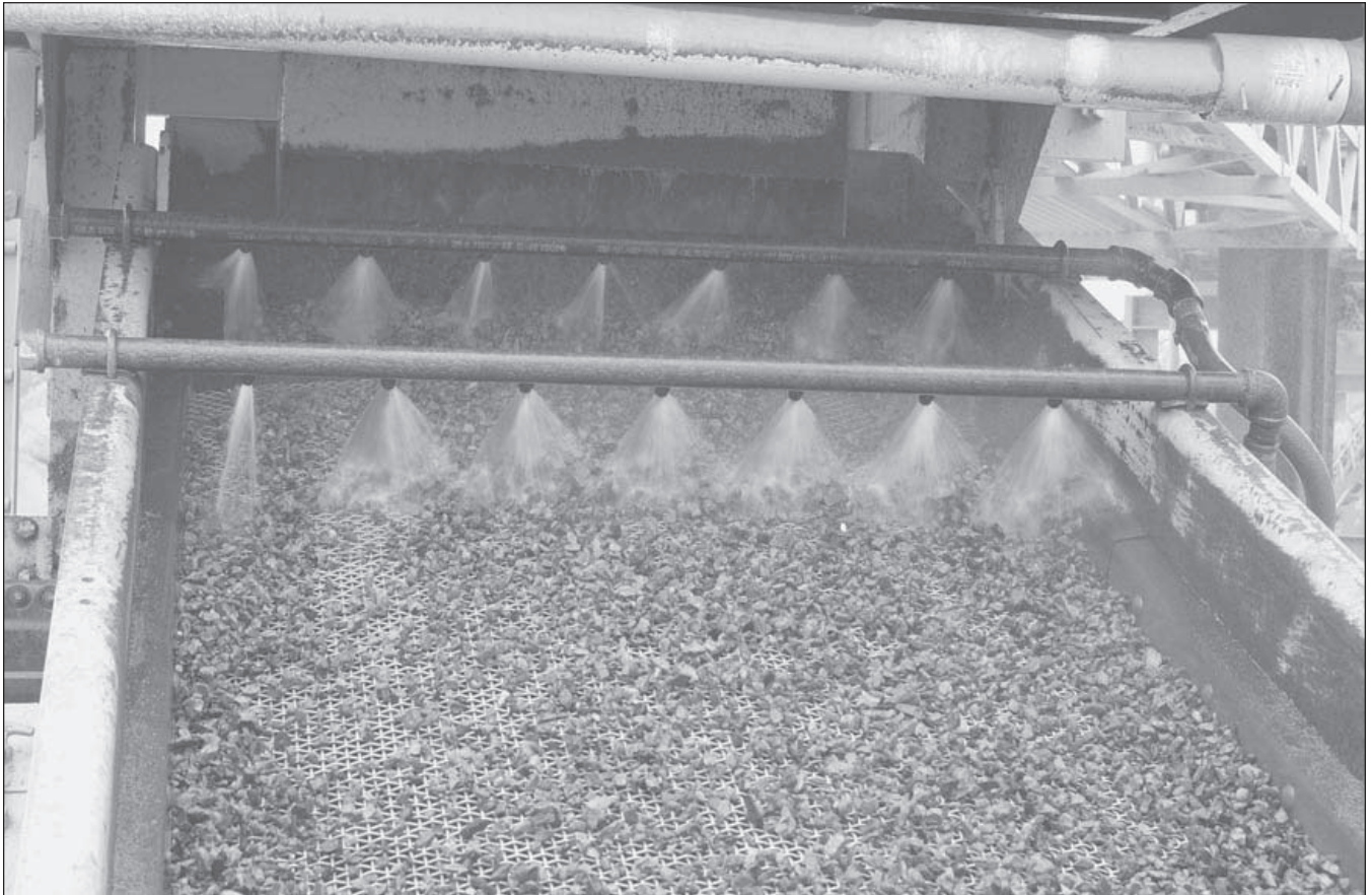
Size no. 8 ( \frac{3}{32} inch to \frac{3}{8} inch) aggregate is washed on the secondary screen at the East Fairfield Coal Co. processing plant in Mahoning County. The no. 8's are double washed to assure quality in the final product.
