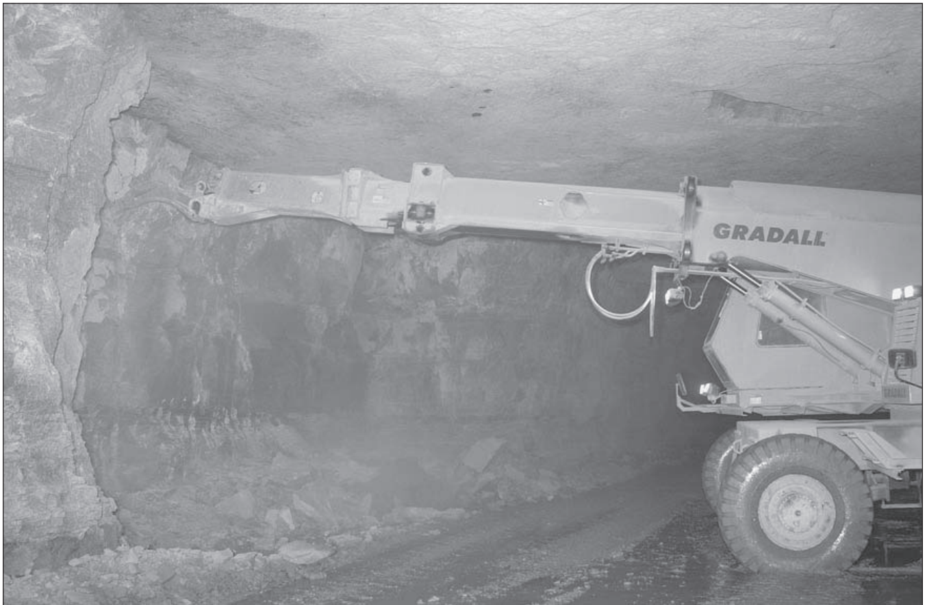
A Gradall XL 5110 scaler is operated by Jason Julian at the East Fairfield Coal Co. underground limestone mine in Mahoning County. The face, ribs, and roof are scaled to remove the loose rock. The scaler follows after the loader has “mucked out” a shot face and the operator has made sure that the room is safe to enter for drilling and loading. The scaler and the roof-bolter make sure that there is no loose rock that may be a hazard to workers.
