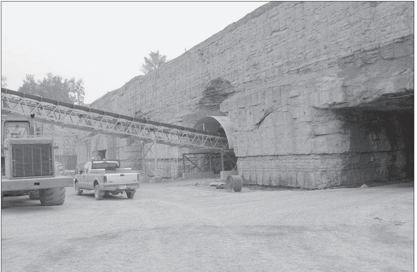
The mine openings at the East Fairfield Coal Co. underground limestone mine in Mahoning County. The entry portal is on the right and the exit portal for the belt carrying aggregate from the mine to the processing plant is on the left.
