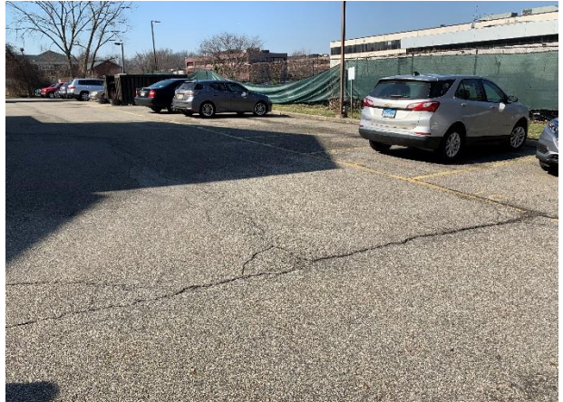
Rear parking lot with cracked pavement.
