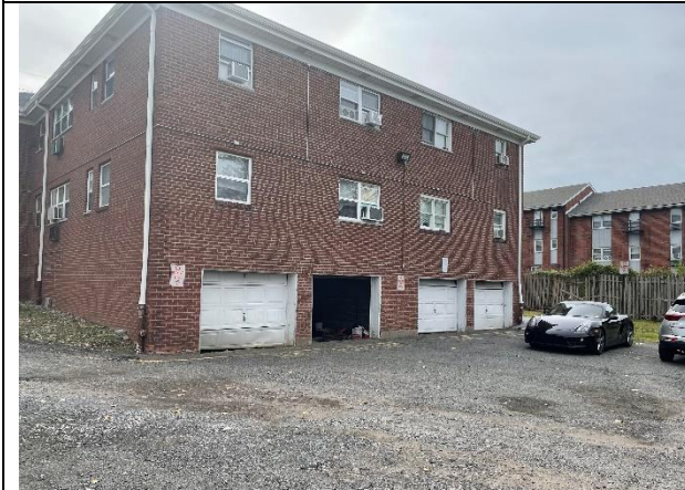
Rear of the building showing the lack of maintenance. Car parked in the fire lane (taken on September 30, 2022)
