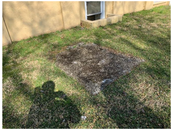
Pavement block in the side yard.
