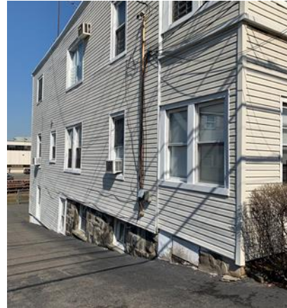
Side of structure with exposed wire and rusted pole.
