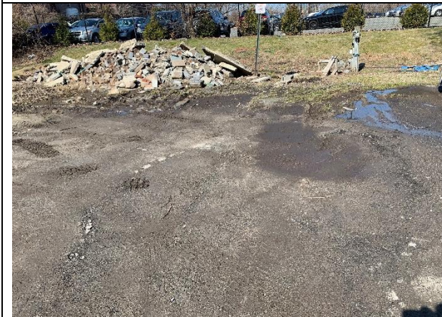
Rear parking area with standing water and storage of broken concrete (taken March 18, 2022).
