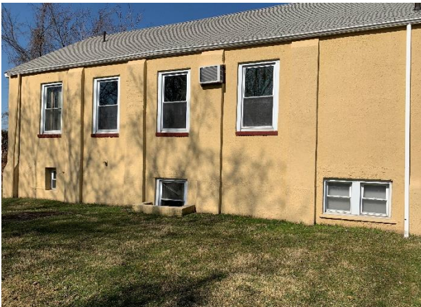
Side of the building with exposed A/C unit.
