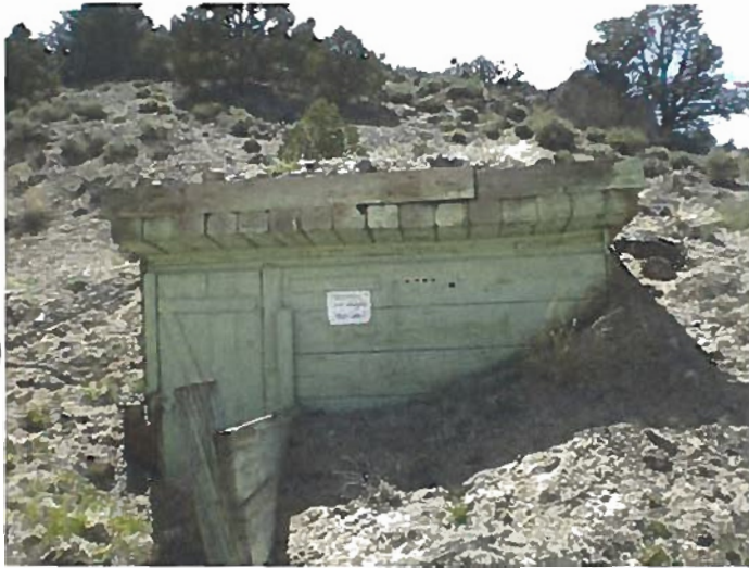
Storage Shed No Longer Used
