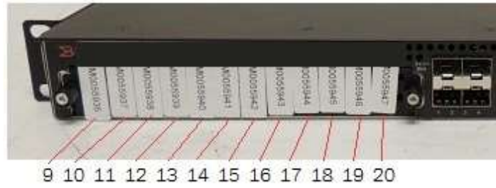
Figure 85 Front view of a Brocade NetIron CER 2024F device with security seals
