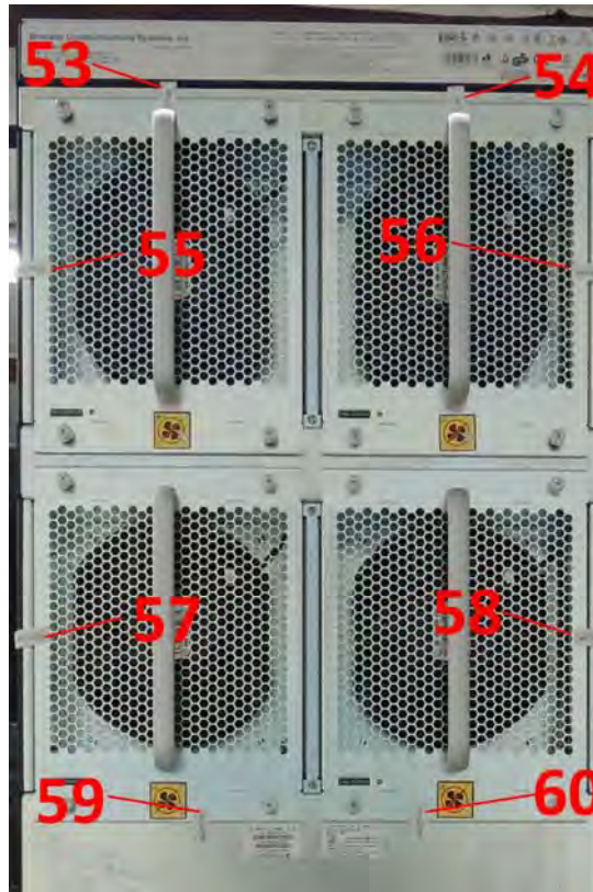
Figure 27 - Back upper chassis of MLXe-32 with tamper labels
