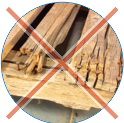
Cracks on the top or bottom boards greater than 1/8" W x 15" L are NOT ALLOWED .
