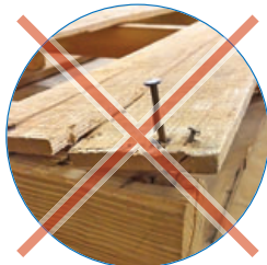
Raised nails greater than 1/8" are NOT ALLOWED .
