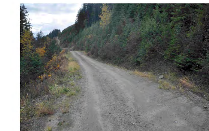
Photo 4. Roads and ditchlines accelerate runoff
