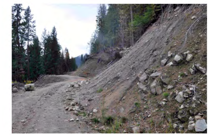
Photo 4. Disrupted drainage from resource roads
