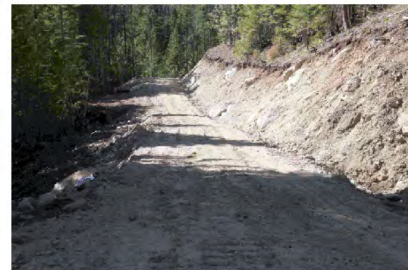
Photo 2. Erosion from road surfaces
