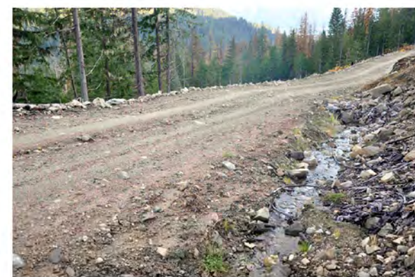
Photo 3. Roads and ditchlines accelerate runoff
