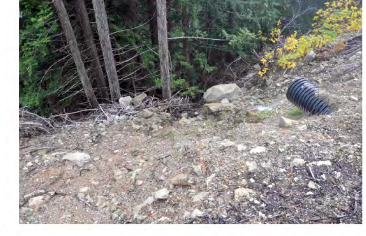
Photo 3. Slope failures from concentrated drainage
