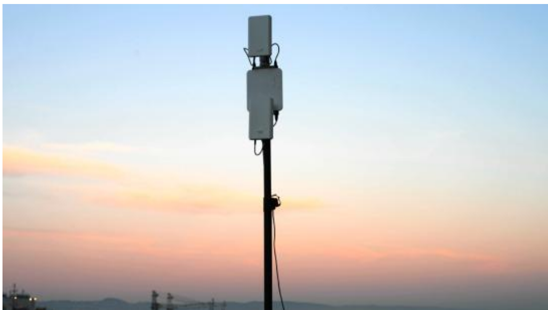
Pole mounted MR66 with Sector antennas, Cisco San Francisco
