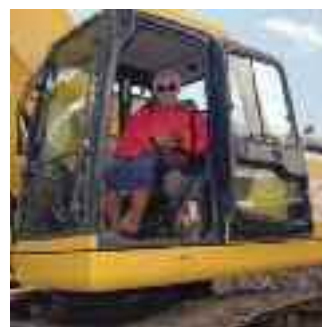
Nancy-Carroll Draper digs the first bucket-load for the Draper Museum of Natural History, October 4, 2000.
