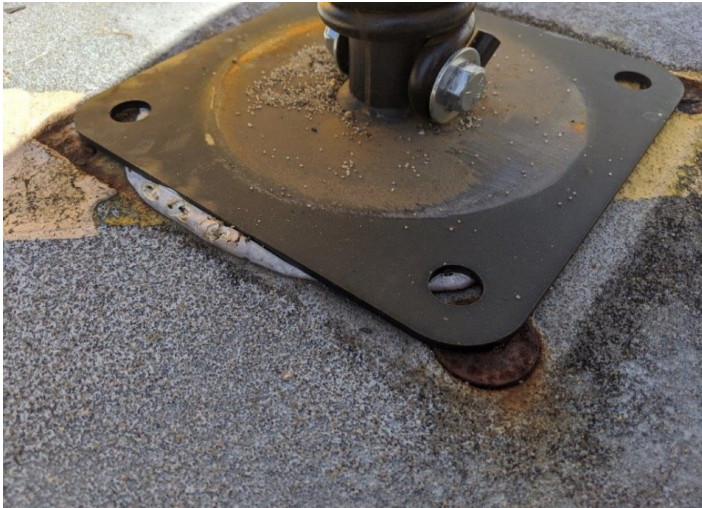
No. 3 View of handicap post base caulking (Sample 3 Rooftop).
