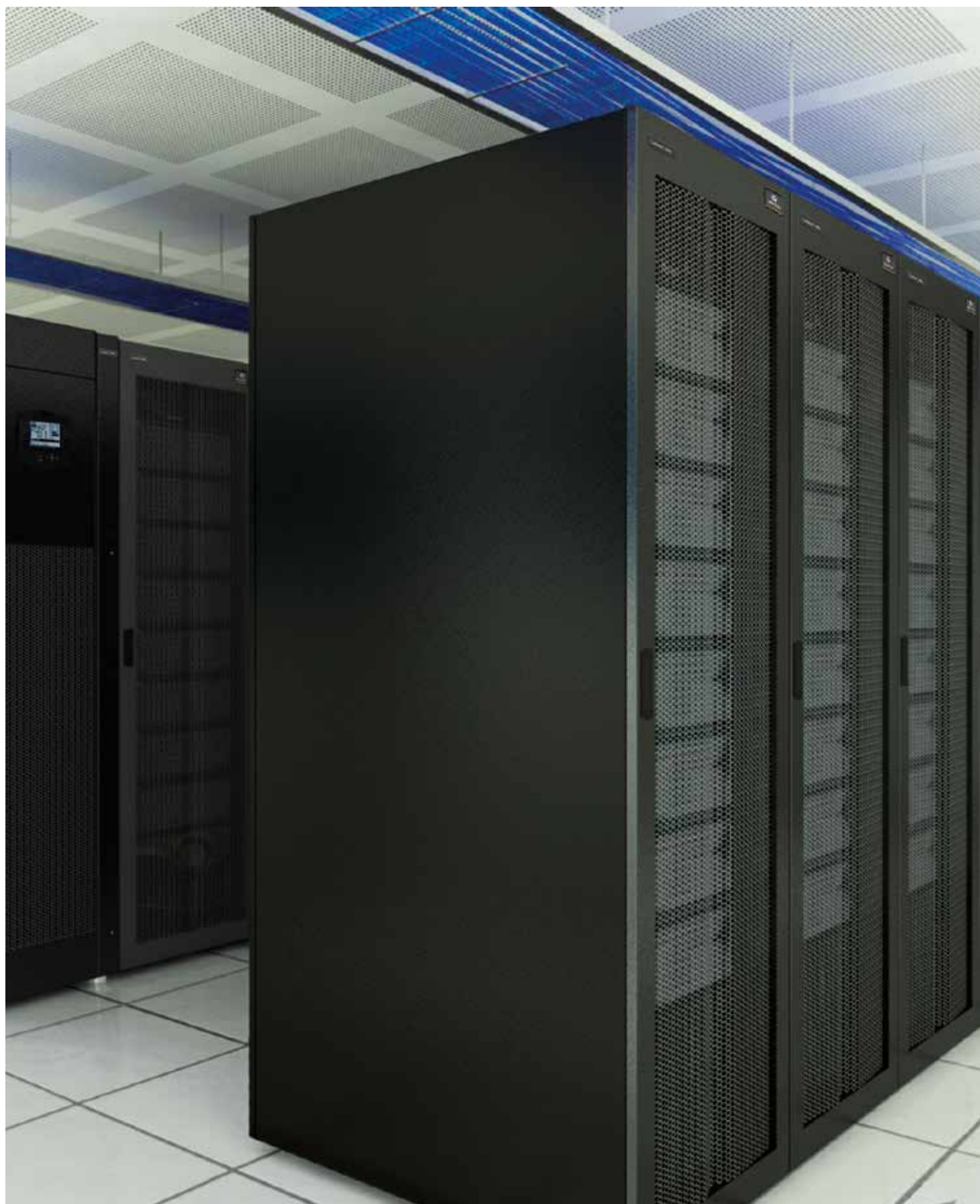
Data center cooling infrastructure for small and large applications.
