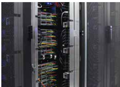
Vertiv™ Knürr® DCM Heavy-Duty Rack server rack for cooling with Liebert DCL, Liebert power distribution modules and integrated cable management
