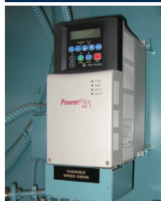
Variable speed drive
