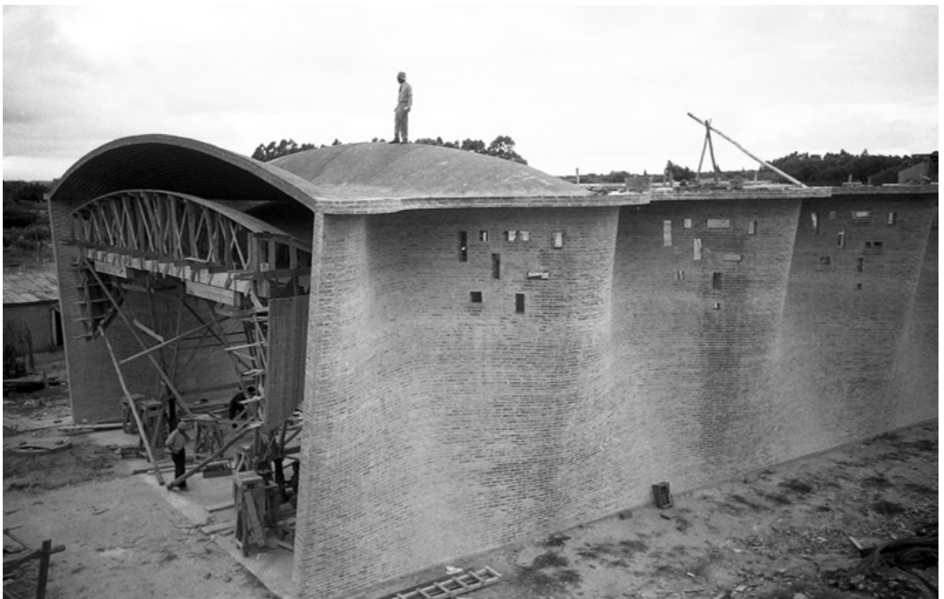
Fig. 2. Church of Christ the Worker, Atlántida, Uruguay, 1958. Eladio Dieste on the roof, watching the dismantling of the scaffolding of the first section of the vault. Dieste & Montañez S.A. Photographic Archive, Dieste Foundation.
