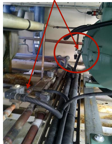
Existing Liquid Injection Supply Piping Re-used
