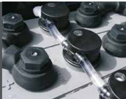
"A-version": automatic mobile filling system on the basis of filler caps and floats. Advantage: all cells are simultaneously refilled in an instant and without spilling up to the right level: time-saving!
