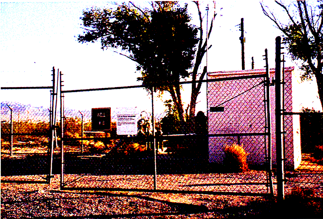
Photograph C-4. Water Well #8, adjacent property to the Water Wells Annex privatization property. View looking north.
