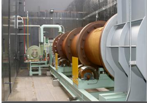
Explosive Waste Incinerator
