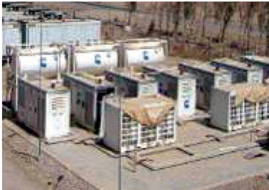
Seven Cummins generators. (Photo provided by USAID)
