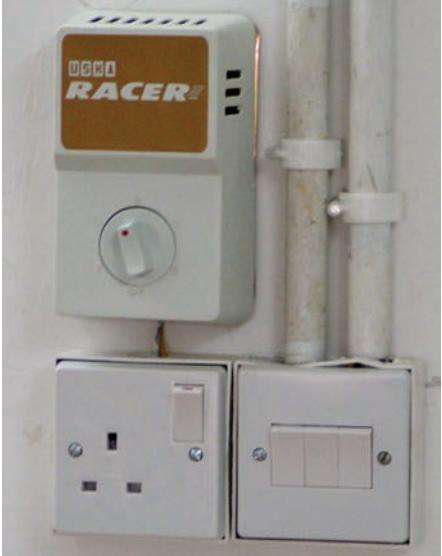
Wiring and components securely fastened to walls.
