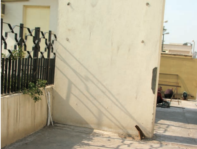
Left side of sally port gate, no locking system for gate.
