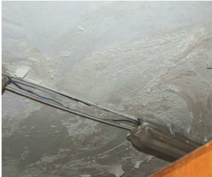
Water damage to the ceiling.
