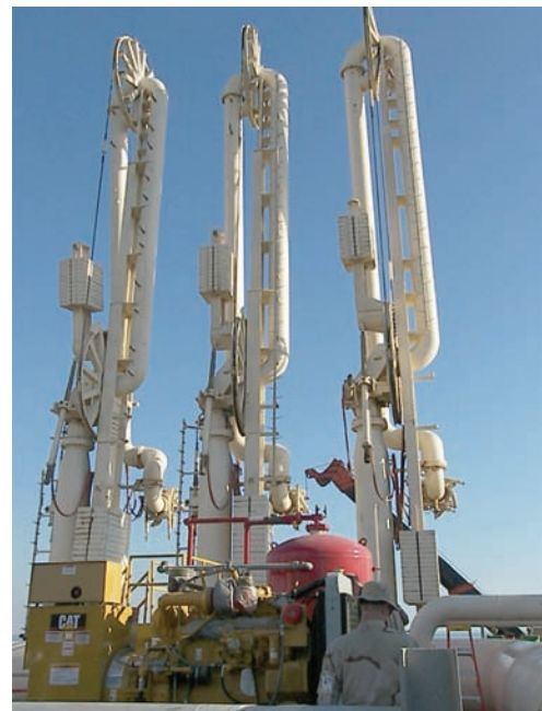
Current condition of refurbished loading arm.
