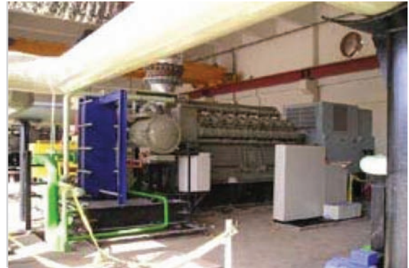
GE generator. (Photo provided by USAID)
