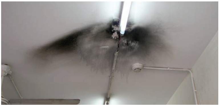
Electrical fire damage around the fluorescent light fixtures.
