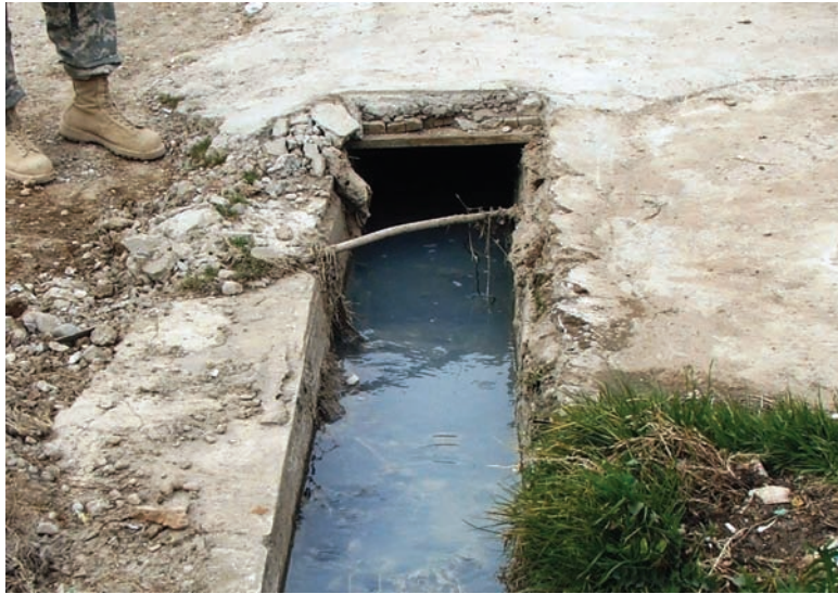
Concrete over sewer culvert was cast too thin, cast without rebar or reinforcement wire and not uniformly mixed.
