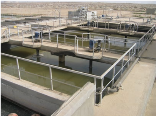
Water treatment remains an important component of the U.S.-funded Iraq reconstruction program.
