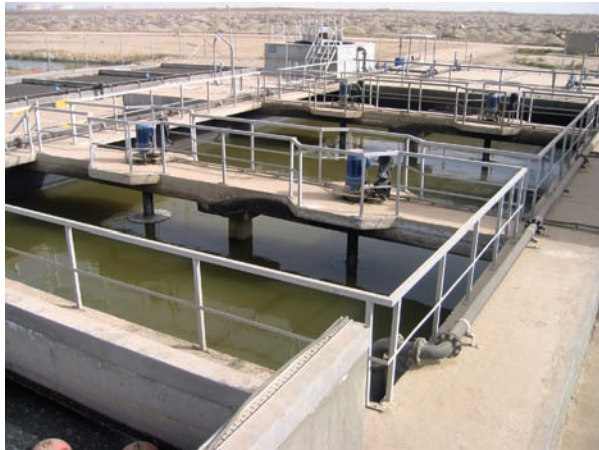
Tallil Military Base wastewater treatment plant.
