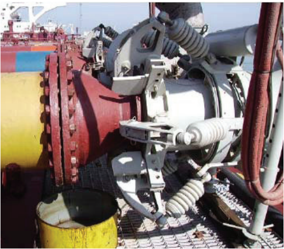
Connection of loading arm to receiving tanker.
