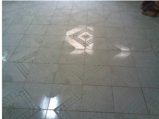
Bathroom floor repair by contractor after SIGIR's inspection. (Photo provided by Westin, Inc.)
