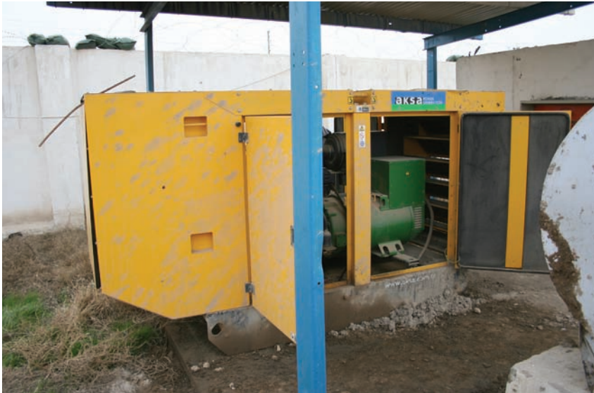
Abandoned generator with no fuel line, low oil levels, broken working-switch gears and controls.
