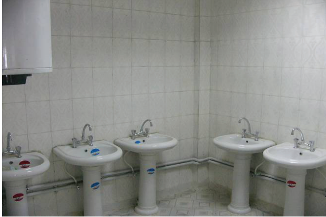
Barracks bathroom sinks and floor shortly after construction was completed. (Photo provided by Westin, Inc.)
