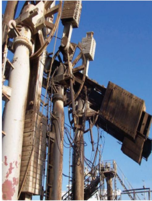
Severe rust, corrosion, and oil leakage of Berth 1 loading arm.
