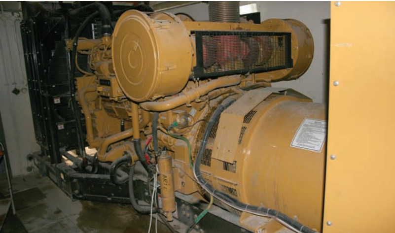
New generator used as a back up.
