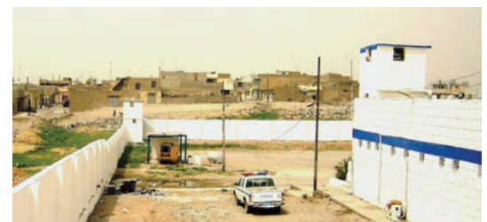
New guardhouse, new generator and fuel tank, new solid block wall and guard tower, and fresh paint.
