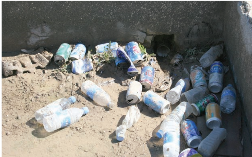
Roof drain blocked by debris.
