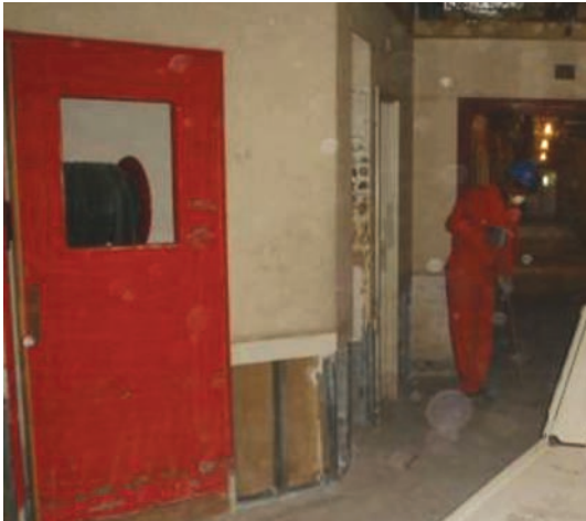
Hallway, water-damaged steel door, and water-damaged gypsum board that had to be removed prior to renovation. (USACE photo, June 18, 2005)
