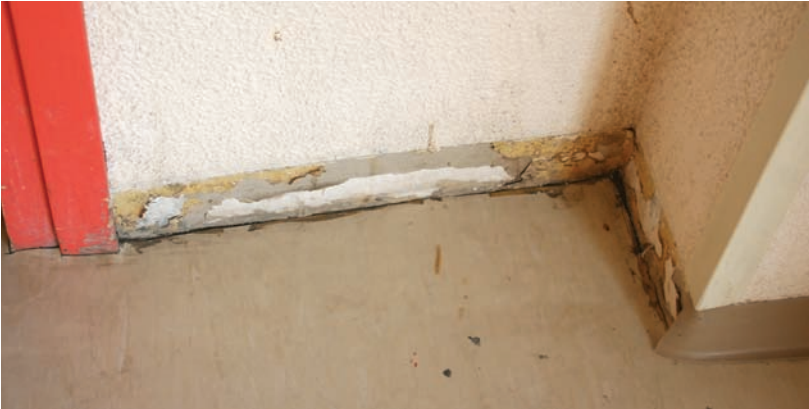
Water saturated and damaged wall with visible mold.
