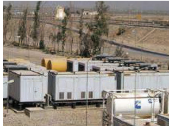
Seven Caterpillar generators. (Photo provided by USAID)
