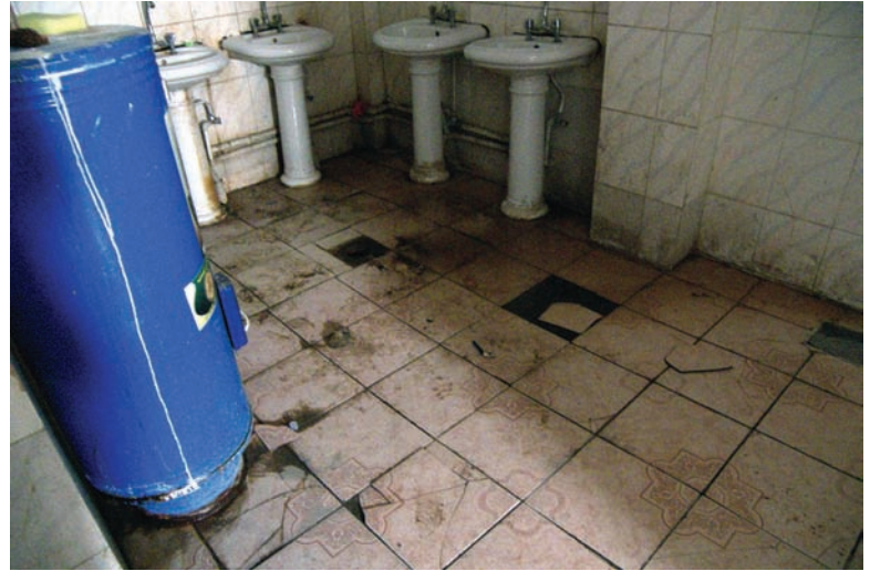
Barracks bathroom sinks and floor at time of SIGIR inspection.
