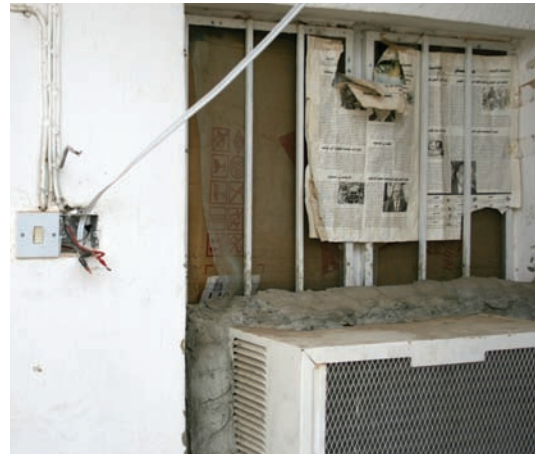
Electrical switch with improvised wirings.
