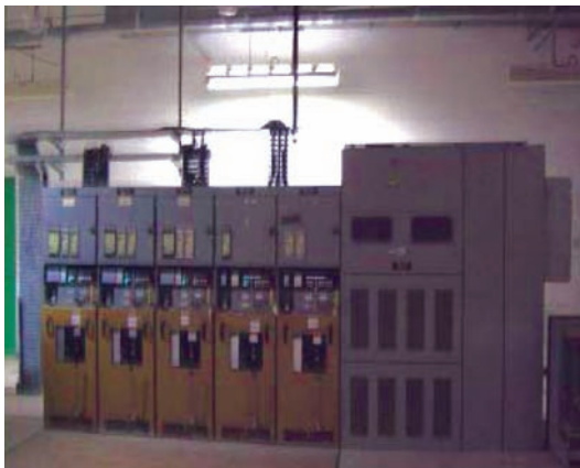
11-kilovolt (kV) system. (Photo provided by USAID)
