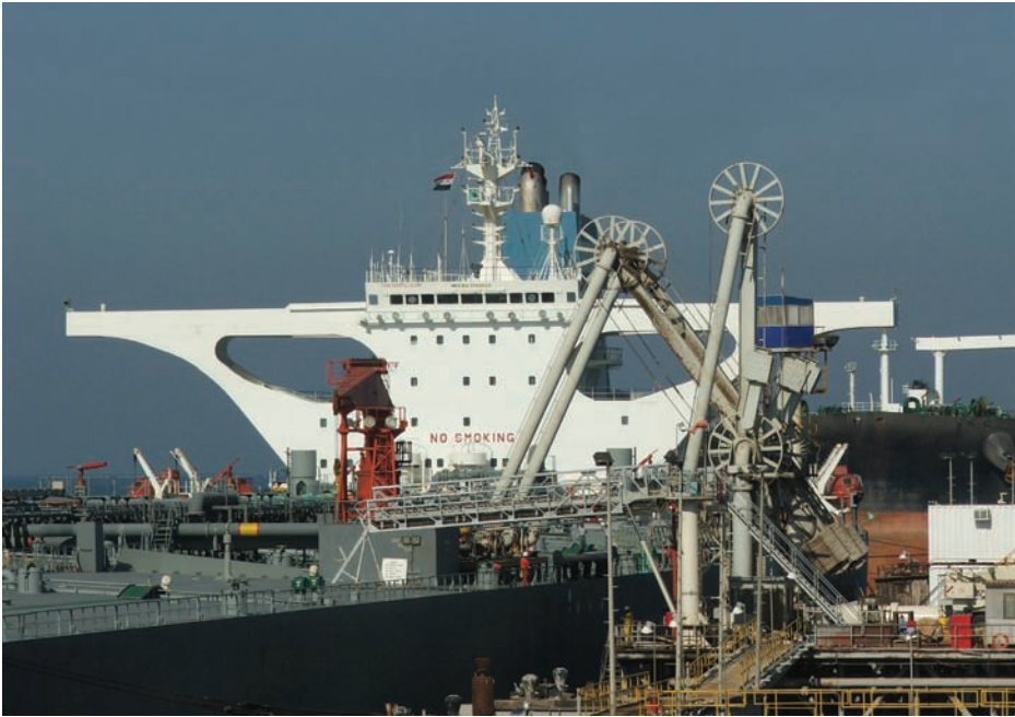
Two loading arms engaged to the tanker receiving crude oil.
