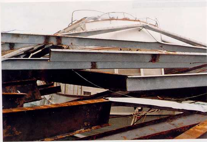
This is how Kalaris looked from the dock. Luckily most of the heavy, black steel girders just missed. All beams had to be cut and lifted before she could be removed.
