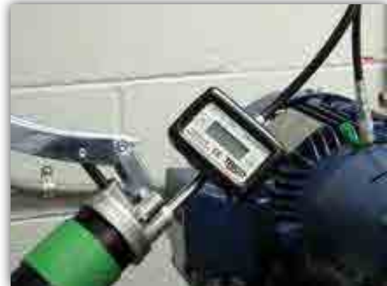
Grease meter being used with Spectrum Grease Identification Products to ensure the right grease goes into the right piece of equipment.
