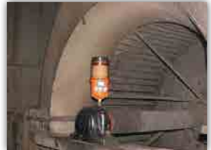
Grease lubricator installed on a blower fan
