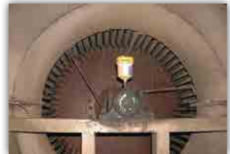
Streamliner V installed on a blower fan
