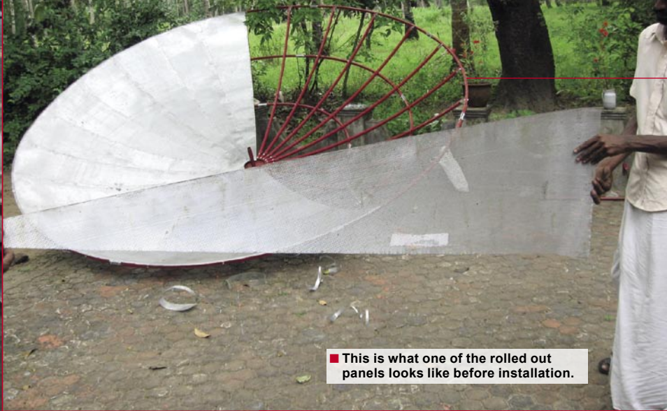
■ The parabolic form takes shape automatically as the wire mesh panels are placed on the frame.
