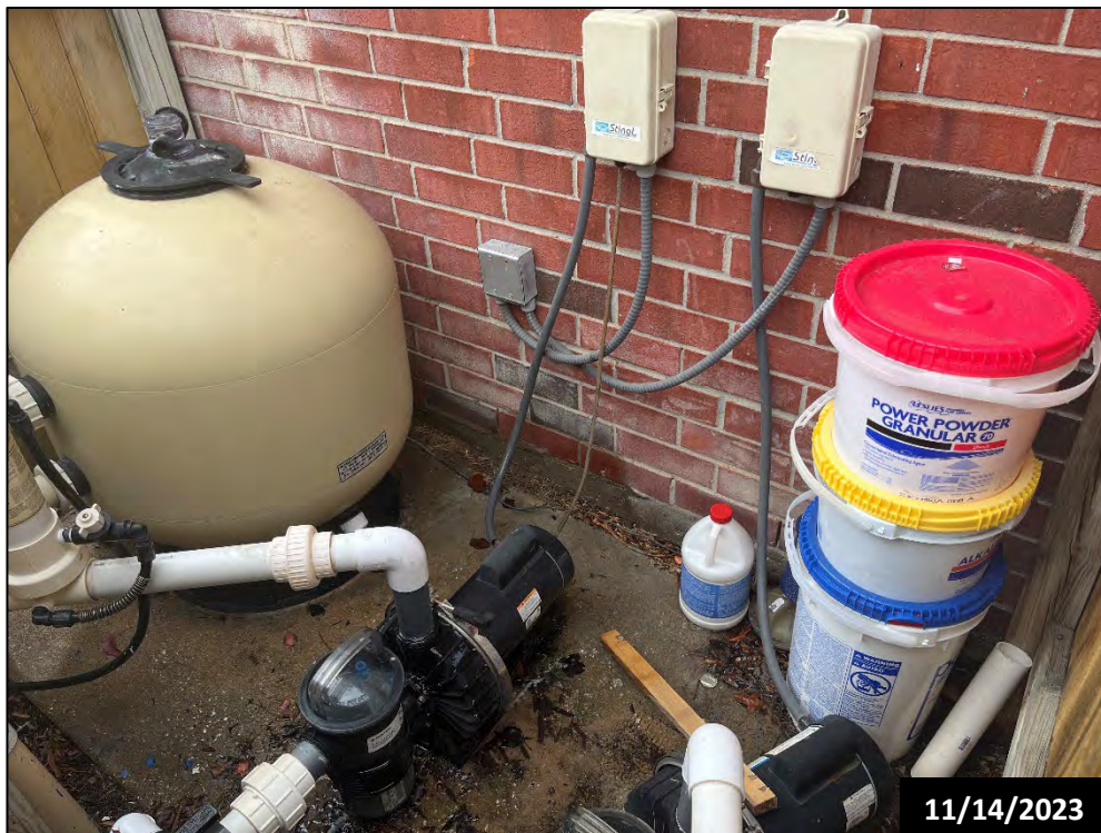
Photo 5) Pool pump equipment and pool chemicals
