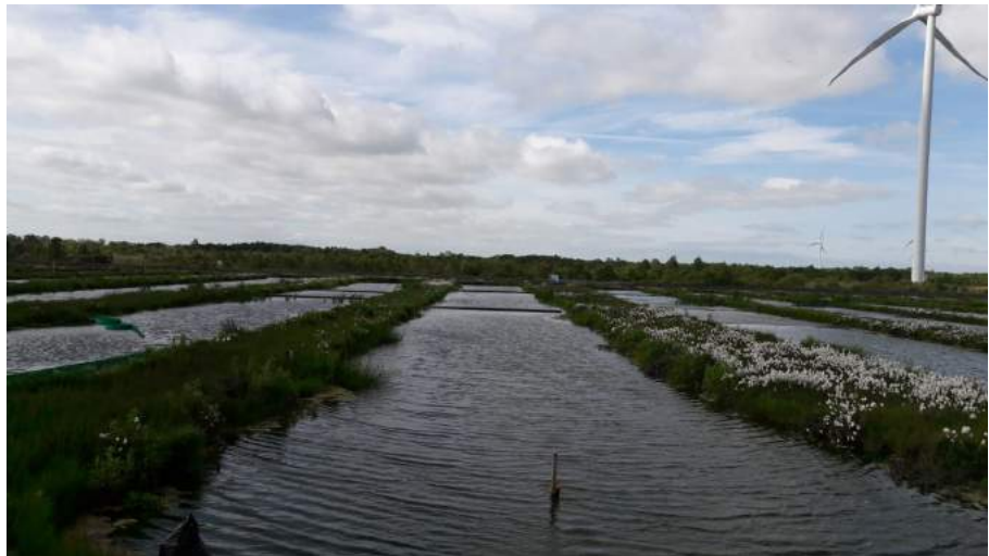
Figure 1: Newly constructed duckweed channels at Mt Lucas fish farm, ready for inoculation with duckweed.
