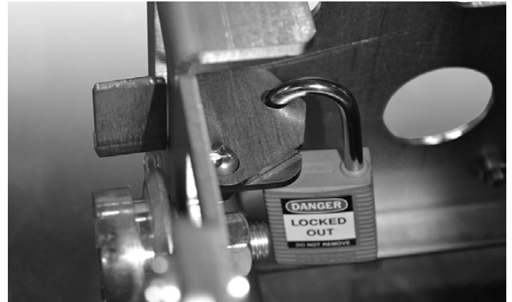
Figure 5.2. Lock-Out Provision (Viewed Inside Breaker Frame)
