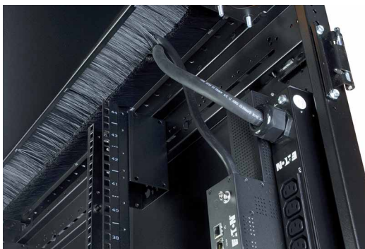
RP Series rack with 2 installed Eaton ePDUs
