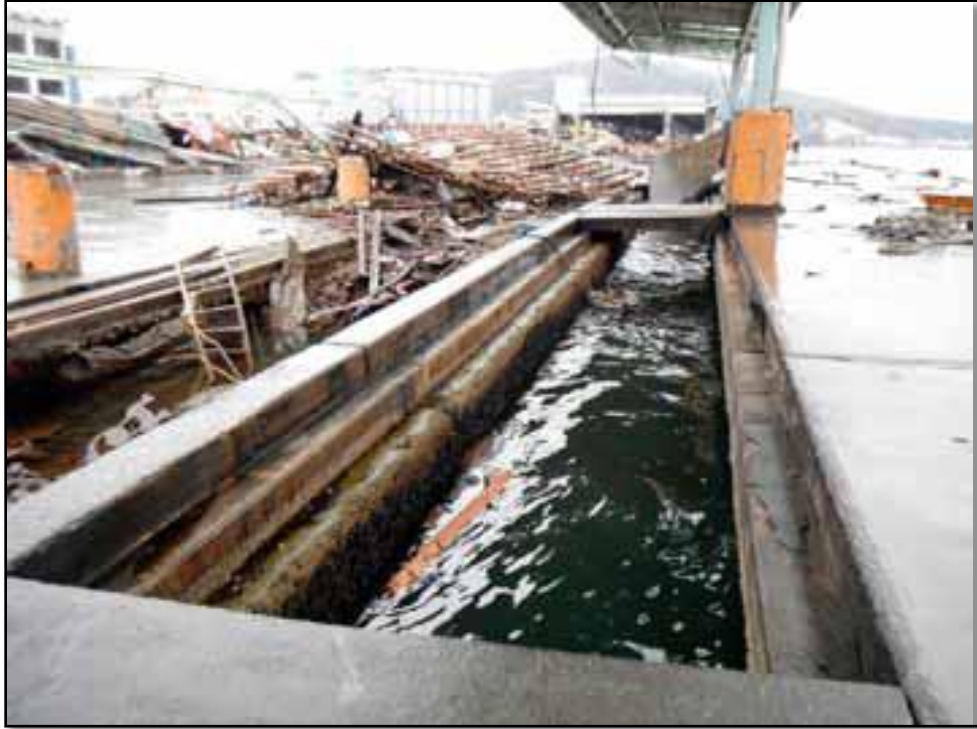
Figure 4-55: Photograph of failed access panels of port in Japan [19]
