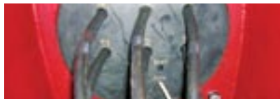
Clearly labeled, separated, and gasketed leads
