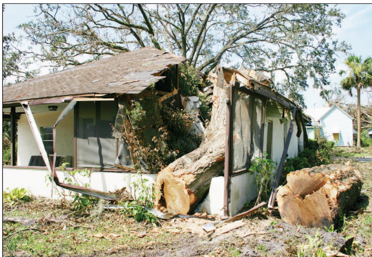
This house was cut in half by a huge oak tree which was uprooted and dropped on it.
