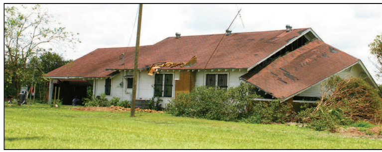
This homeowner lost some roofing and an entire wing of the house parted company with the rest of it.
