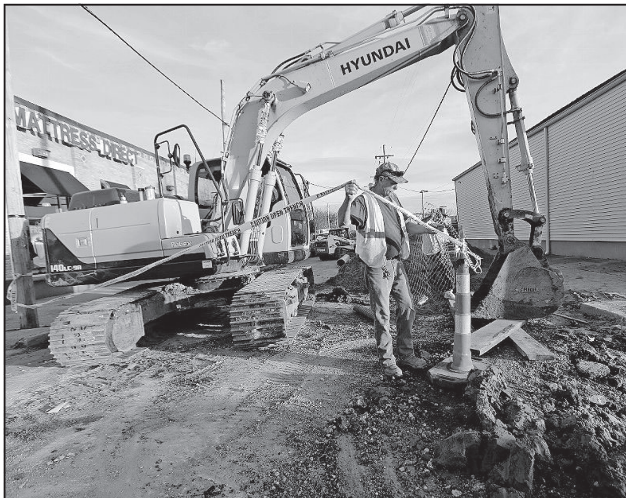
Workers fix a sewer main below the sidewalk Jan. 31 in Mid City New Orleans. [GERALD HERBERT/THE ASSOCIATED PRESS]
