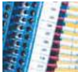
Terminal Block Labels
