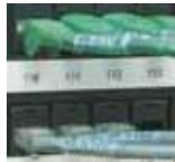
Patch Panel Labels
