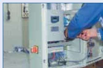
Control panel with frequency in inverter
