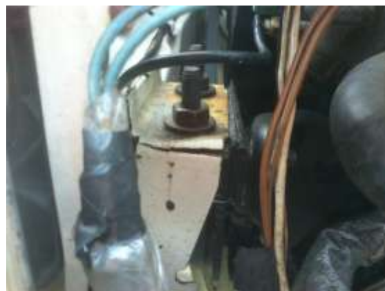
Cracked front mount
