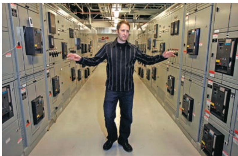
Opus Interactive CEO Eric Hulbert in the main power room in his growing downtown data center that will eventually consume enough electricity to power 150,000 homes.
