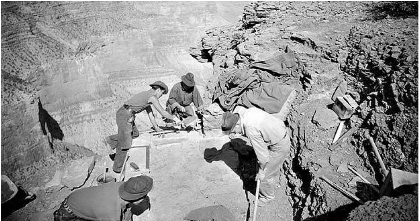
Figure 6. Civilian Conservation Corps (CCC) constructing the in situ Fossil Fern Exhibit along the South Kaibab Trail during 1937 (NPS).
