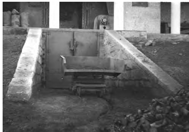
A hopper wagon on the short section of track at the rear of the Willoughby Incinerator during construction of the refuse hopper (behind camera) on 17 July 1934. David Warner Collection, Willoughby District Historical Society.
