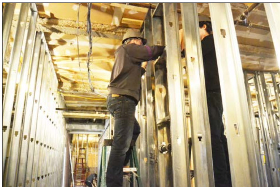
Cabinet, electric and plumbing students from Bay Path have been working on a 7,700-square-foot space at the Webster High School, building new administration offices.
