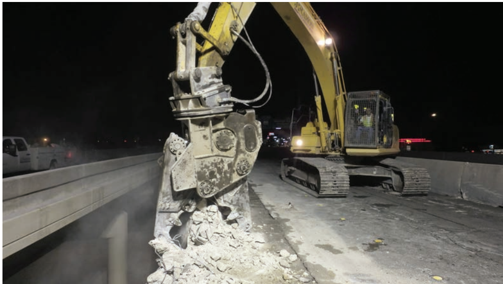
JR RAMON used an 80,000-pound Komatsu PC360 excavator with a CAT pulverizer attachment to demolish the 3-foot-tall, 1-foot-thick, rebar-reinforced concrete rails.
