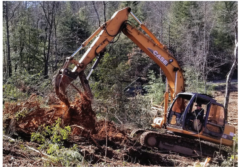
Brian Thompson is not only splitting and harvesting stumps, but also digging trenches for silt fence, loading log trailers, and backfilling stump excavations with a Ransome Shark Tooth RST 150 Stump Splitter/Harvester mounted on a CASE CX160 Hydraulic Excavator.
