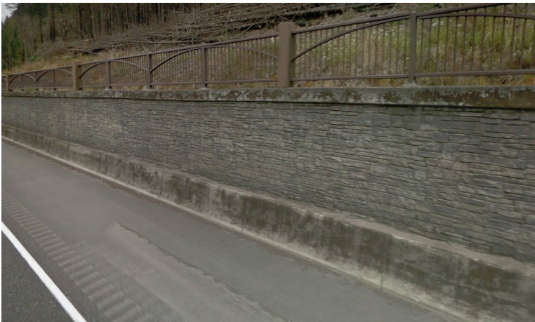
Figure 21: Photo of existing MSE Wall on John B. Yeon section of the HCRH State Trail adjacent to eastbound I-84.
