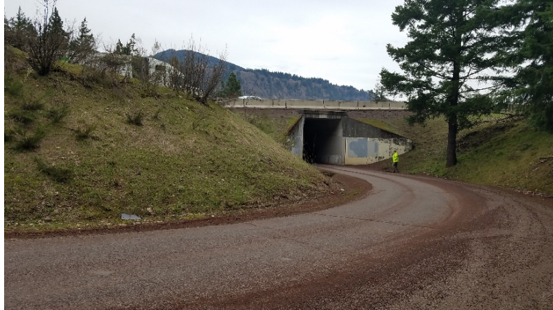
Figure 15: Looking Northeast at the East End of Segment F Mitchell Point Undercrossing of I-84
