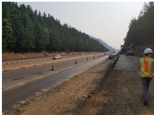
Figure 2: Construction of HCRH State Trail between Wyeth and Lindsay Creek in August of 2018.
