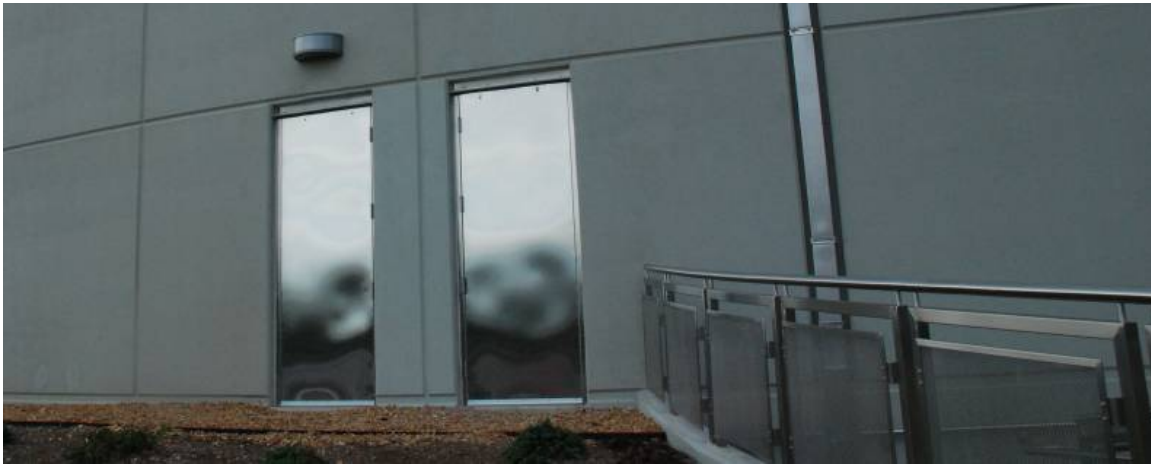
Figure 3-5 Emergency Exit Doors
