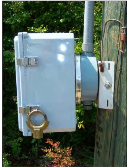
SWITCHED BANK CAPACITOR CONTROL
