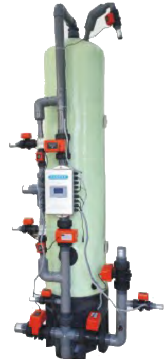
Mixed bed control system
